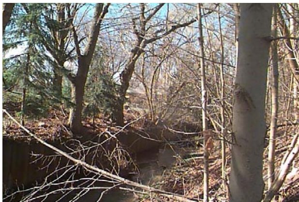
Figure 1. Existing condition of Consolidated Drain # 1
